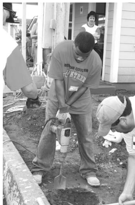
Above: Beckman Coulter volunteer, Michael Sharpe, uses a jack hammer to help speed up work on the project
